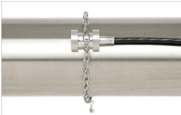
PT100 transducer fixed to pipe
