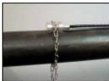
PT100 sensor fixed to pipe
